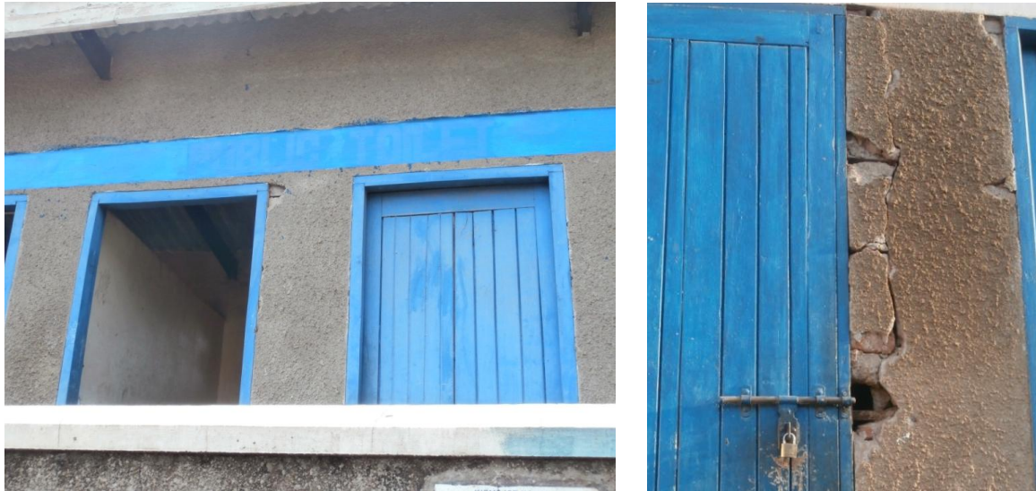
Figure 11 Different degree of wall erosion
