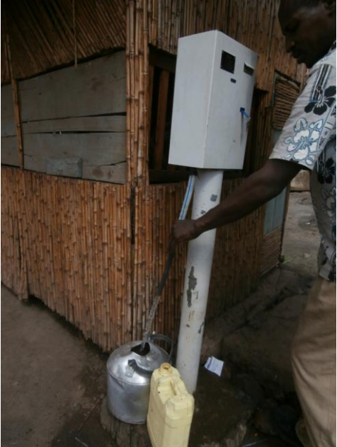
Figure 14 Relocated pre-paid meter in Katwe I
