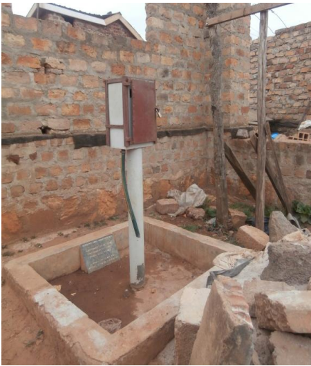
Figure 15 Protected pe-paid meter in Bwaise III
