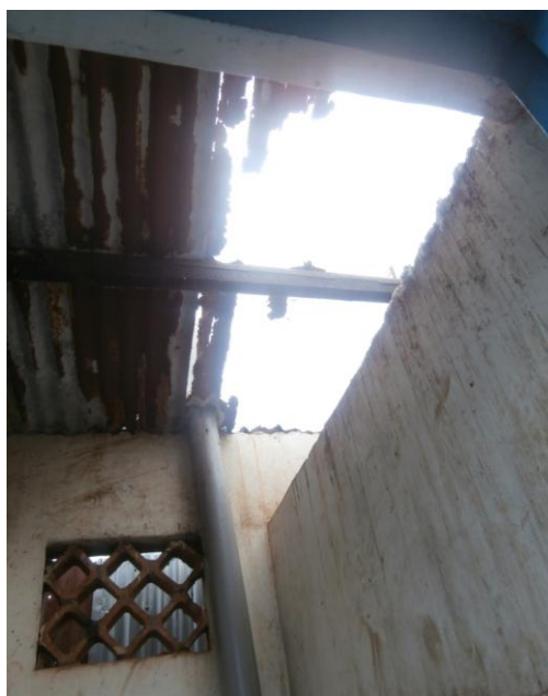
Figure 12 Roof damage of public toilet in Kisenyi II
