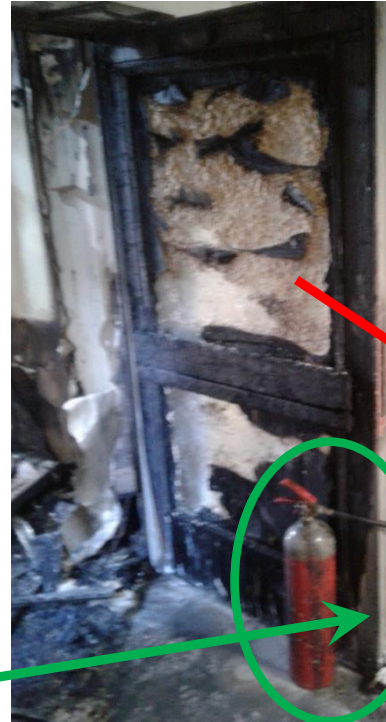
Fire door on side of flames
