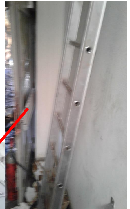
Fire door on the "safe" side
