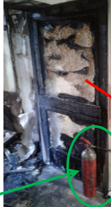
Fire door on side of flames
