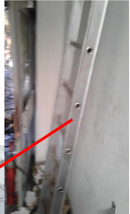
Fire door on the "safe" side
